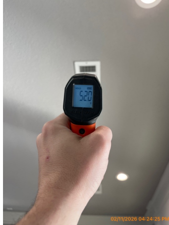
Downstairs main supply
