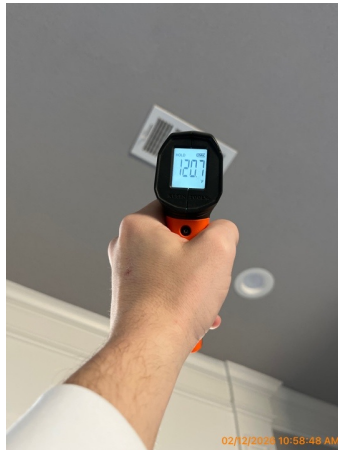
Downstairs main supply
