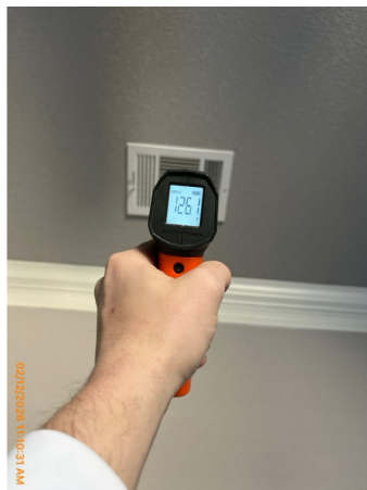
Downstairs back right bedroom supply
