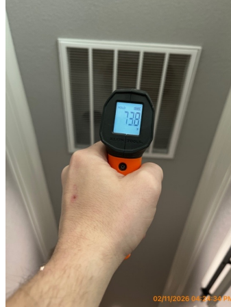
Downstairs main return
