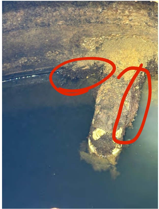
Roots in tank
